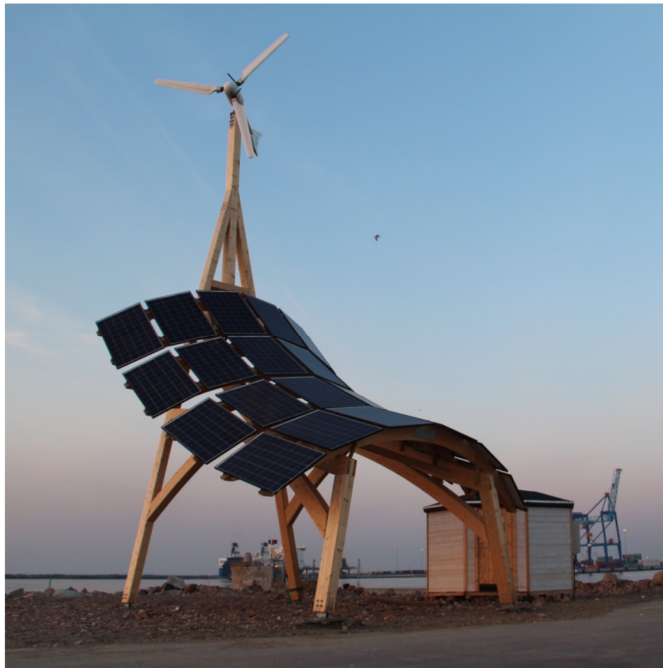
Figure 1: Giraffe 2.0 Hybrid Wind-Solar Power Station
